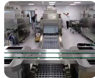
Flight conveyor with lowered entry section and waste management
