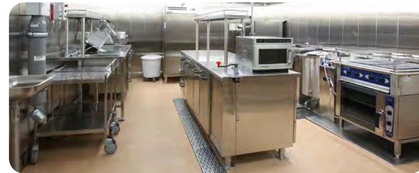
Layout, design and delivery of equipment for galleys and laundry
